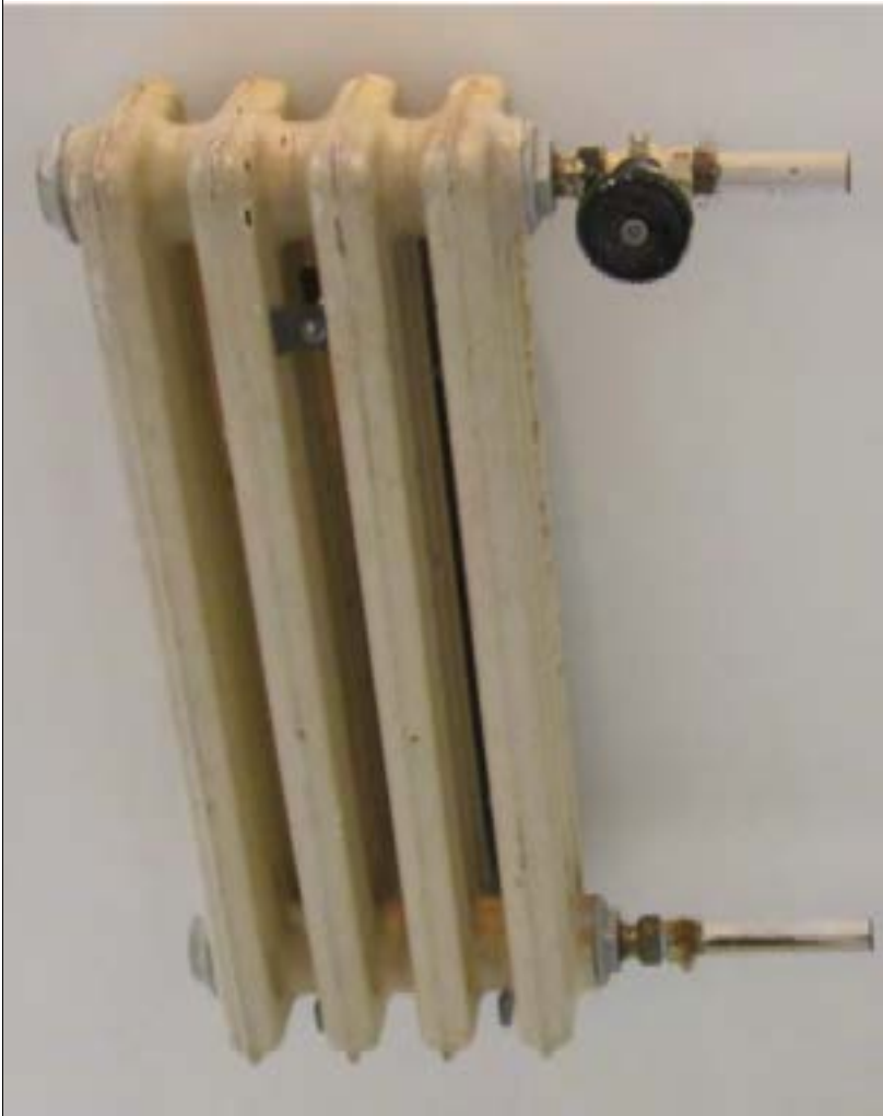
Traditional cast-iron radiator
