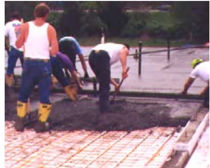
Notice where the tubing is in this 6" heated concrete slab
