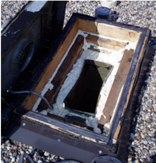
Air seal at curb below fan
